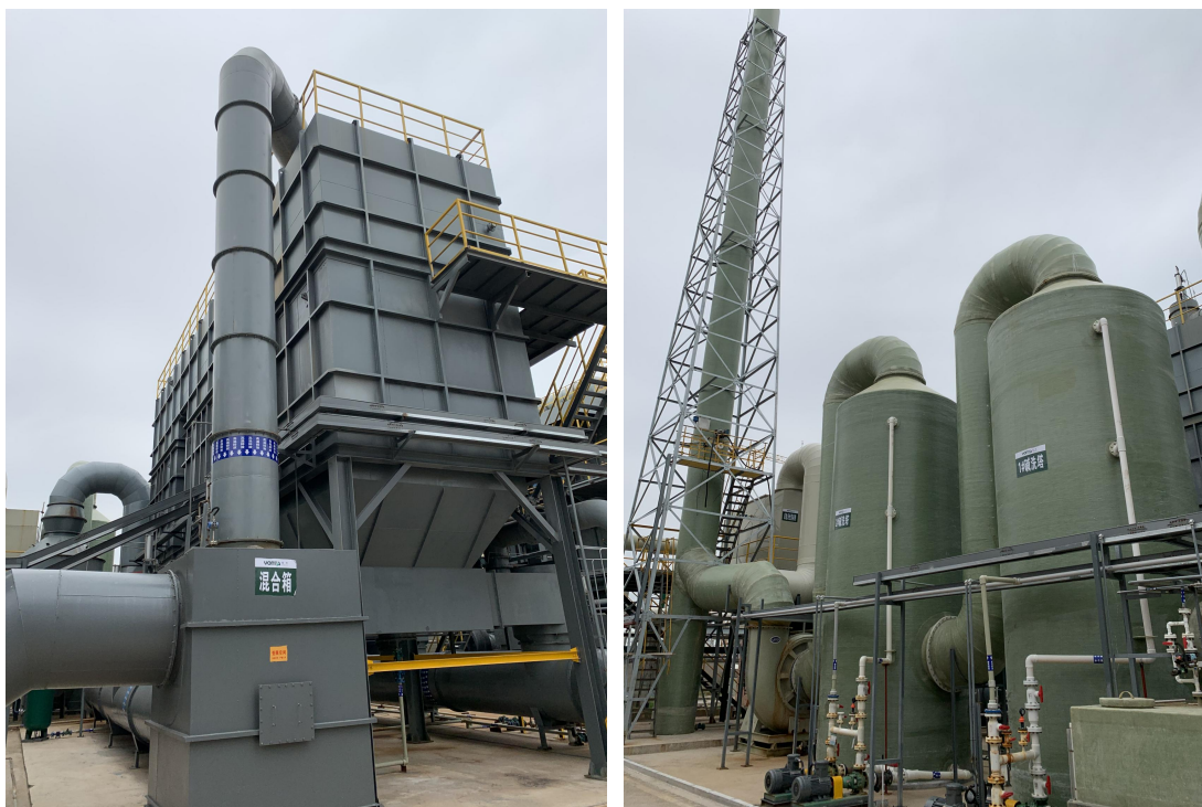
“碱喷淋+RTO+二级碱喷淋”设施及其排气筒
